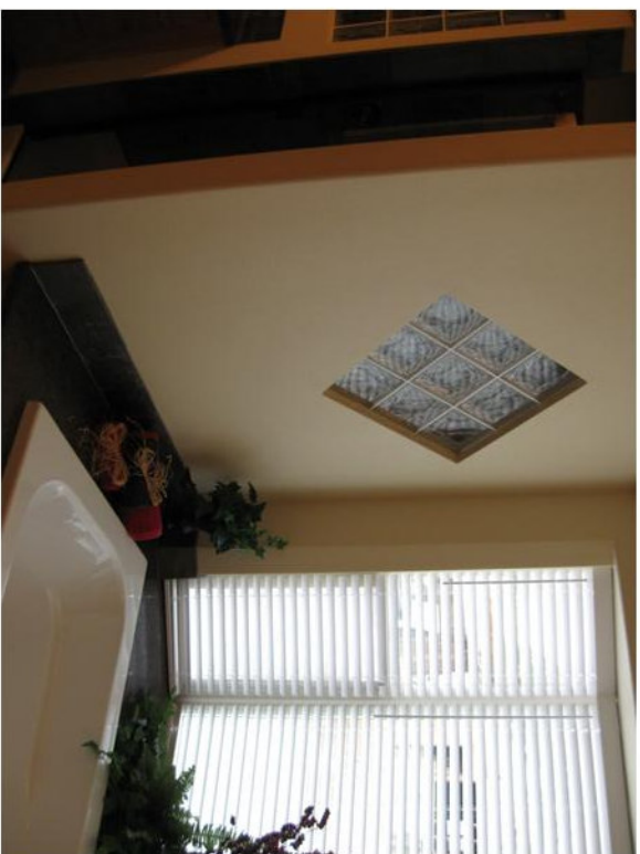
Decorative glass blocks in shower stall adding natural light into shower and a touch of elegance to the appearance of the bathroom
